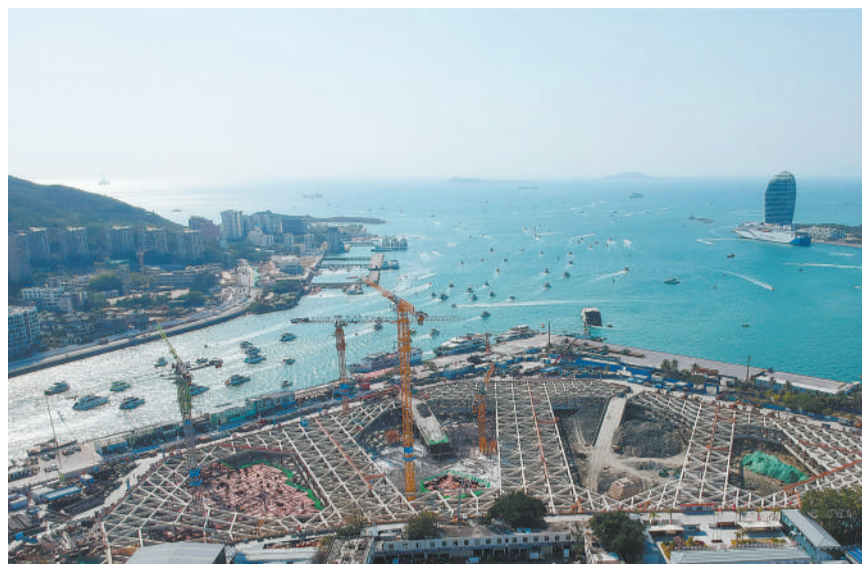
The Hainan International Cultural Relics and Artworks Exchange Center and the Hainan International Cultural Exchange Center are under construction in Sanya city. (PHOTO: XINHUA)
