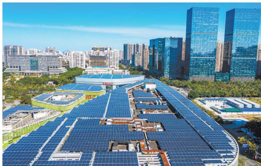
Photovoltaic panels installed on rooftops of the Riyue Square in Haikou city, Hainan province. (PHOTO: VCG)
