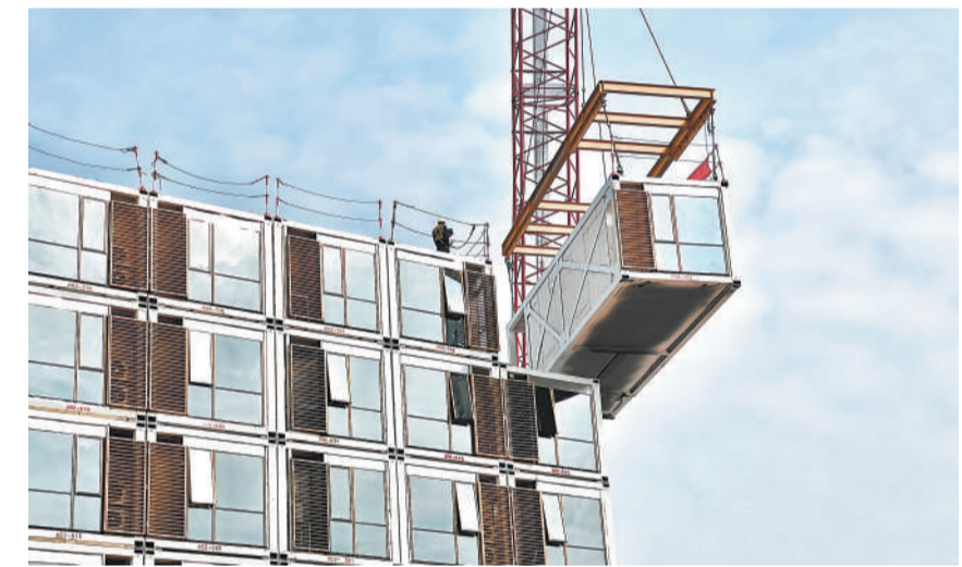
Pre-made steel structures are assembled at a construction site in Huizhou, Guangdong province. (PHOTO: VCG)
