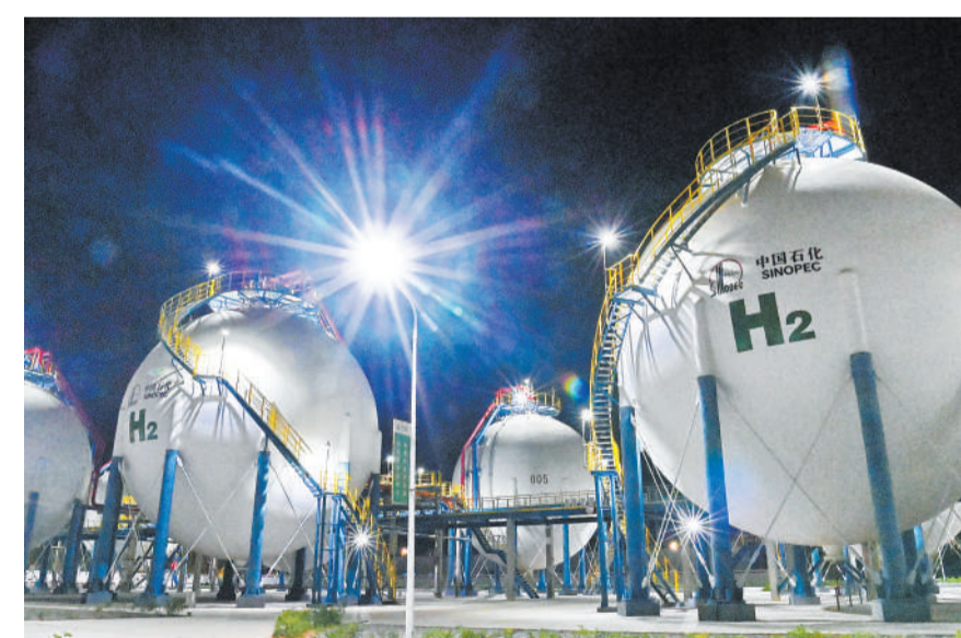
Hydrogen storage tank installation area in Aksu, Xinjiang Uygur autonomous region. (PHOTO: VCG)
